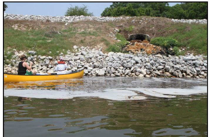
Wastewater outfall from the South Lagoon into the Leaf River.
